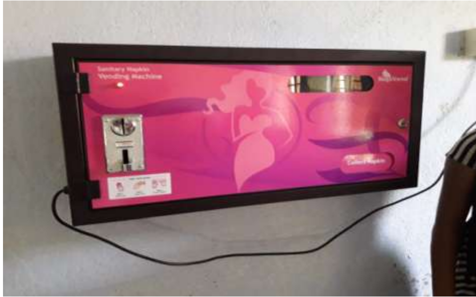
Installation of Sanitary Vending Machine inside girl's common room.
